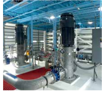
The water treatment facility for the city of Venice, FL, features pump motors from Nidec/U.S. MOTORS. Project details at https://watercollaborativedelivery.org/project/venice-water-treatment-plant/ Photo courtesy of Haskell https://www.haskell.com/
